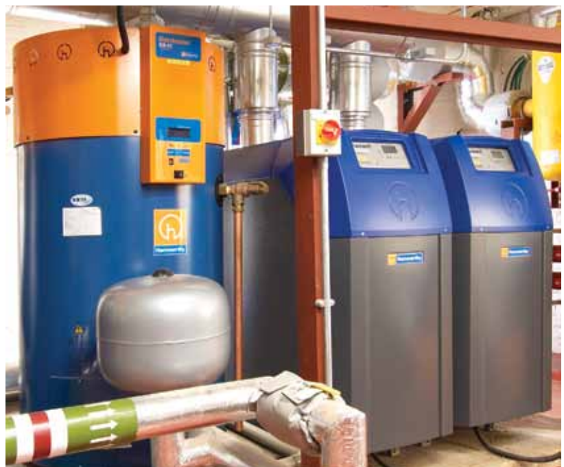
Purewell VariHeat high efficiency condensing boilers with a Dorchester DR-FC condensing water heater.
