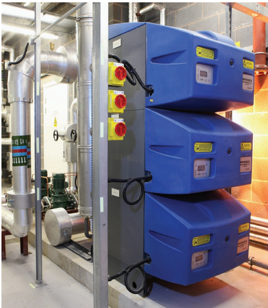
Wessex ModuMax boilers
