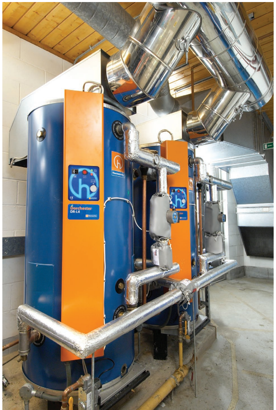
Dorchester DR-LA water heaters supplying all domestic hot water requirements
