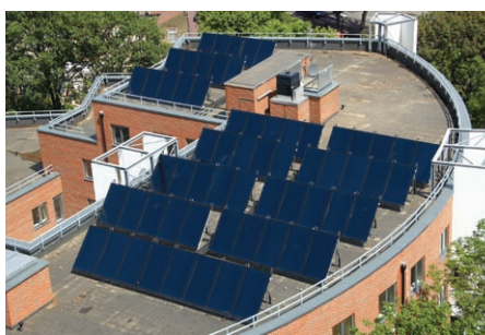
Hamworthy solar collectors at work
