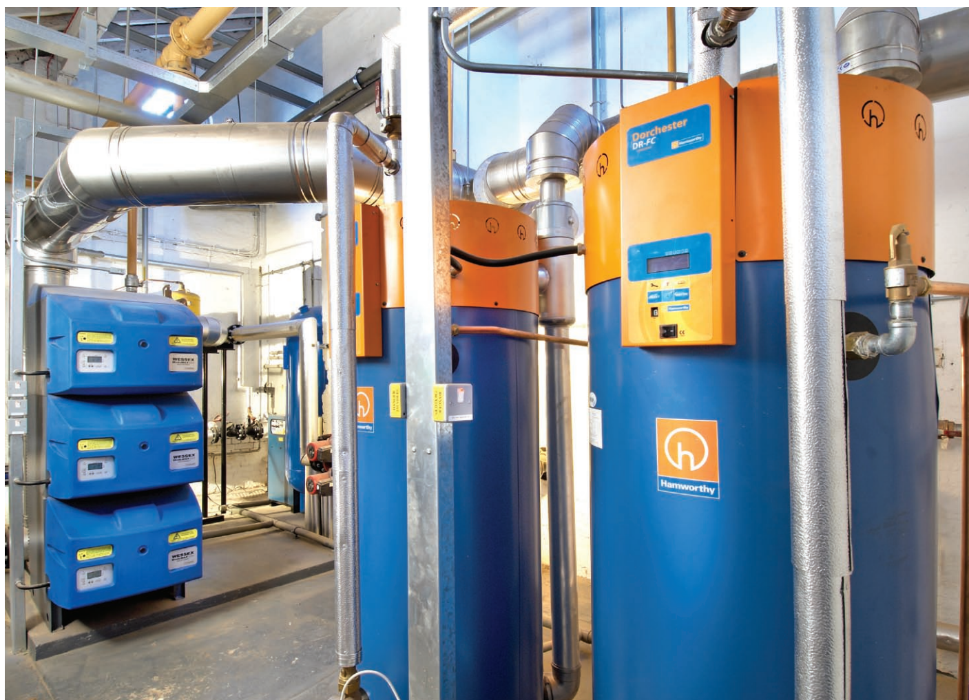
Saving space with Hamworthy boilers allowed two water heaters to be installed
