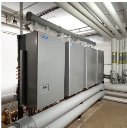
Milborne wall hung boilers
