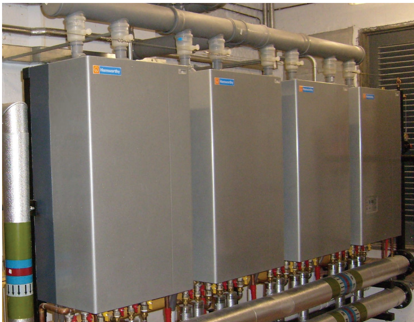
Four Milborne boilers working in unison to heat the busy Cathedral and lower energy costs
