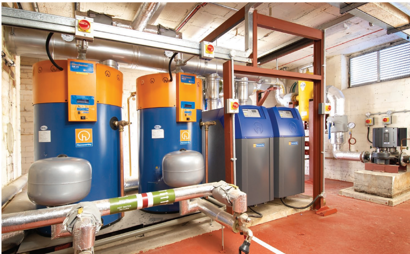
Hamworthy Dorchester water heaters and Purewell VariHeat boilers working in unison to provide heating and hot water
