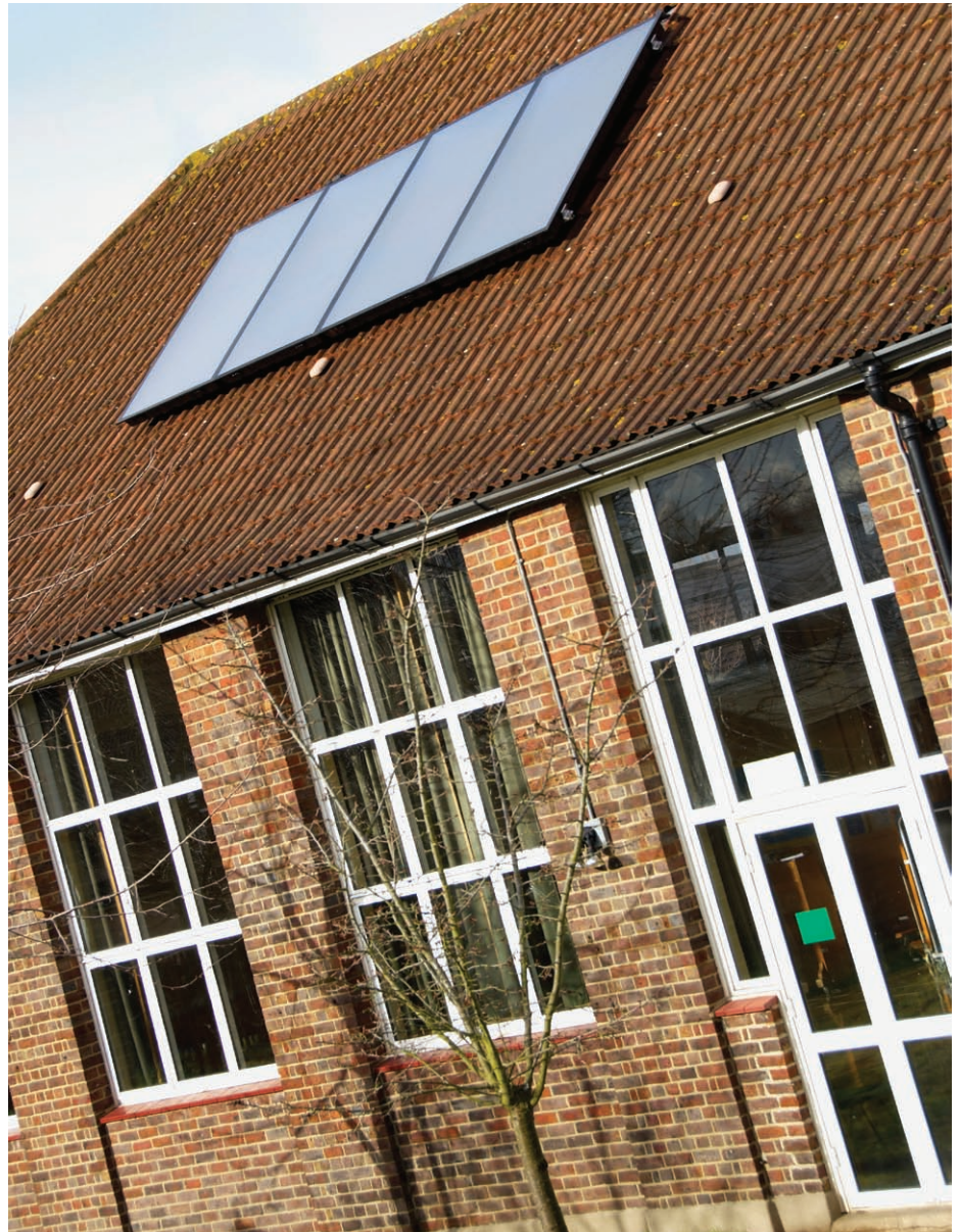
Hamworthy high efficiency solar collectors
