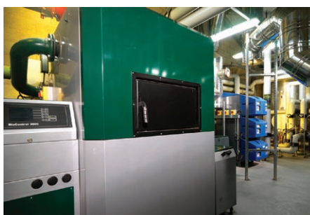
Wessex ModuMax boilers supporting biomass
