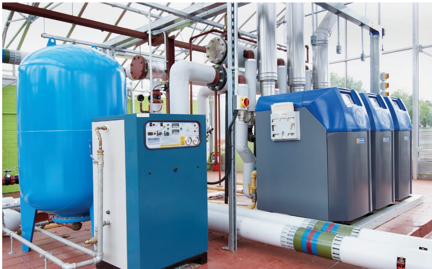
Hamworthy products at work ensuring optimum growing conditions for the nursery's plants
