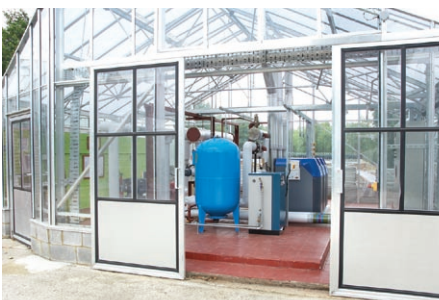
The greenhouse plant room
