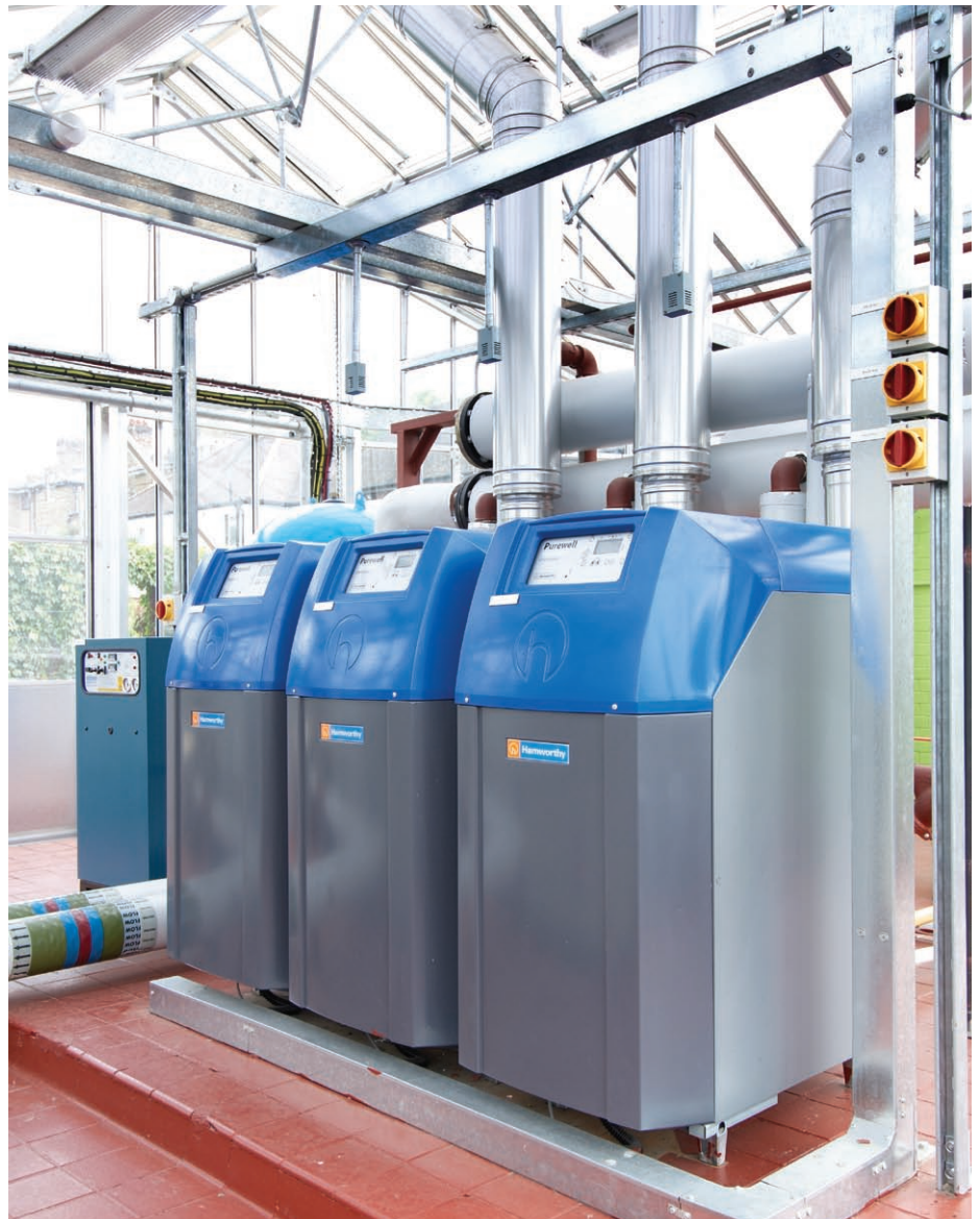
BMS compatible Purewell VariHeat boilers are ideal for West Ham Nursery
