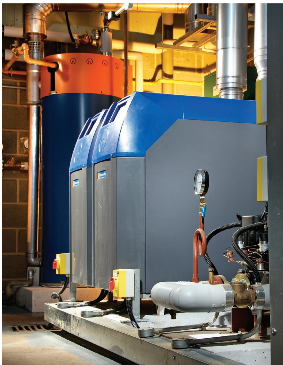
Purewell VariHeat boilers and a DR-FC water heater at work
