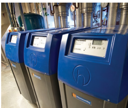
Purewell VariHeat boilers at work
