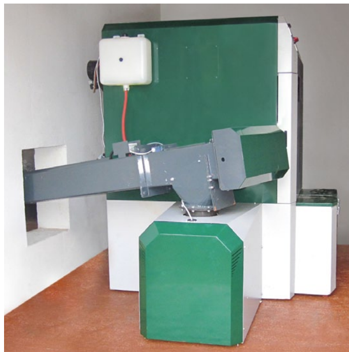
Firematic boiler with rising fuel feed auger and drop chute above the intermediate hopper, and a water tank for the burn-back protection sprinkler.
