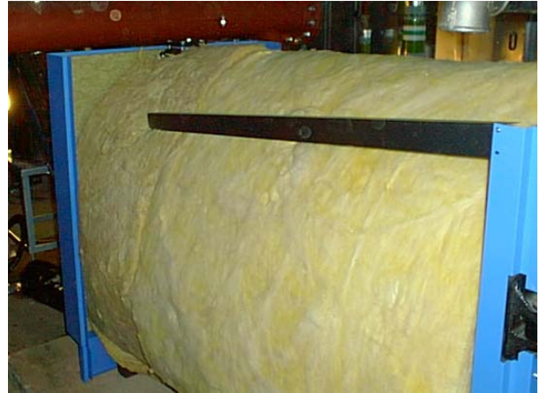
Picture 5: Boiler Body Insulation
